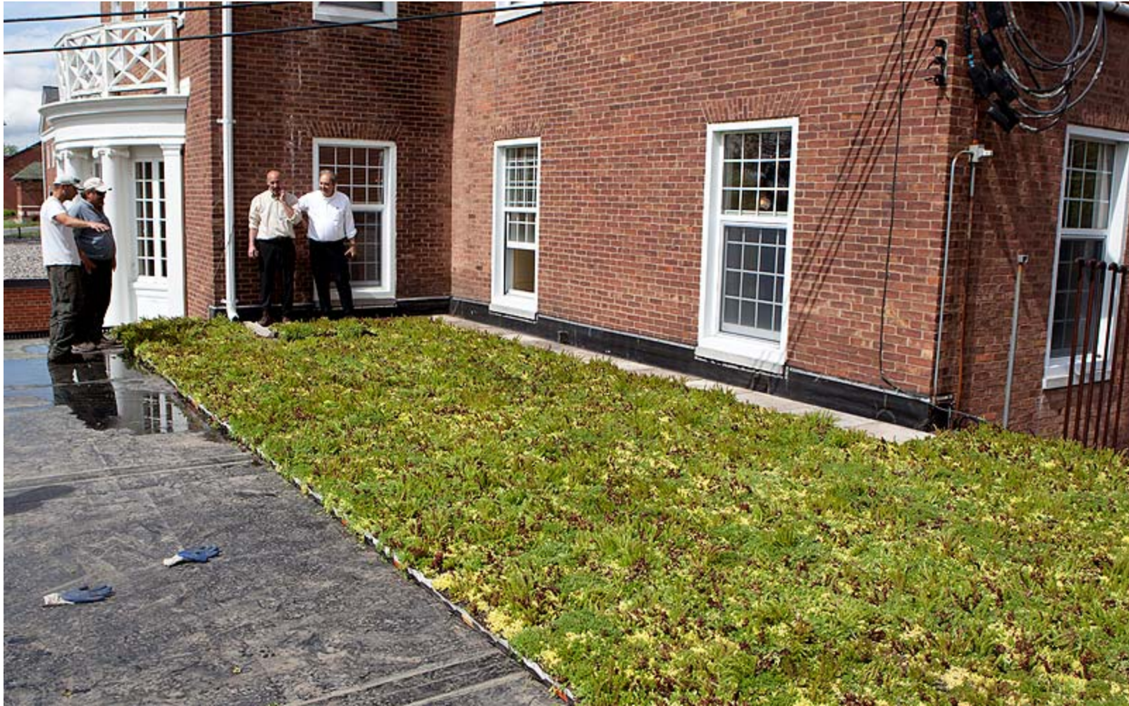
Buildings and Grounds staff meet with contractors who are installing a green roof on Comstock Hall. The pilot project was initiated by the Climate task force as a means to help with storm water management, reduce the heat island effect, and improve the insulation in the new Comstock renovation. (2011)
